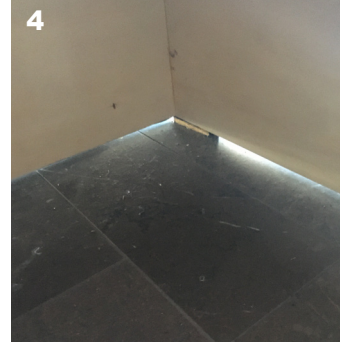
4 The wall is not hermetically sealed at the bottom, which can cause drafts.
