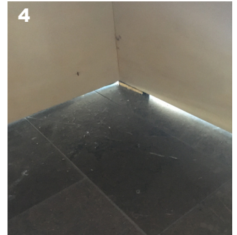
4 The wall is not hermetically sealed at the bottom, which can cause drafts.
